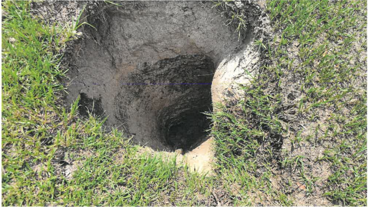
Site Photo No. 3 – Surface Depression in DRA 8 located at Indigo East South in Ocala, Florida
