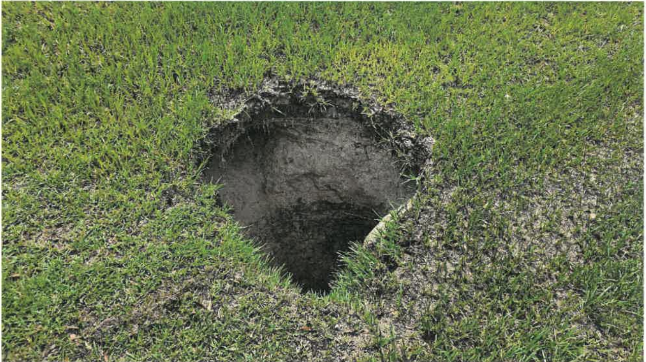
Site Photo No. 2 – Surface Depression in DRA 8 located at Indigo East South in Ocala, Florida
